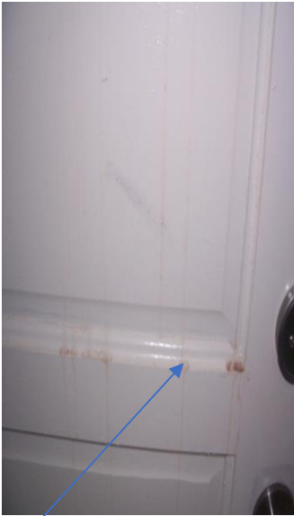
Water seeping through the wood.
