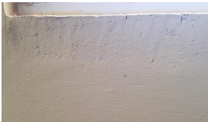
Unfinished walls in kitchen
