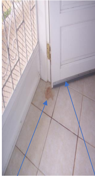
Water accumulates at bottom of door.
