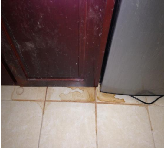
Water leaking under the kitchen sink
