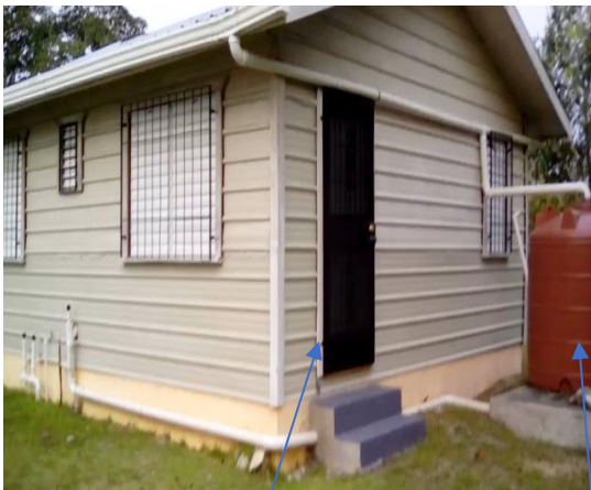
This is the rear of the building. I purchased a vat and installed a second door with bar. Had Ben followed our directions, we would not need a new vat. I paid him because he said he bought one and installed it, but he did not.
