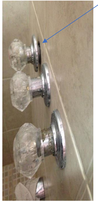
All faucets were loosed and had to be sealed.
