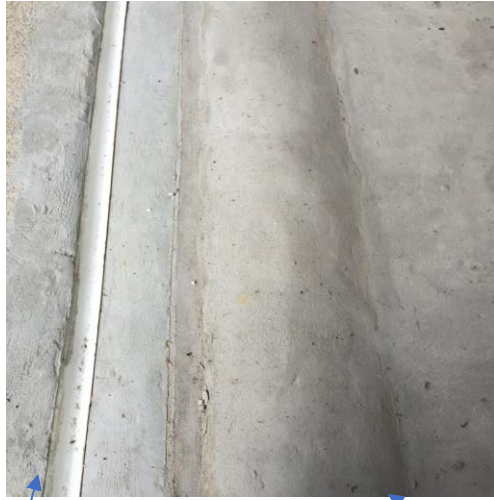
drain outside garage door bump inside garage
