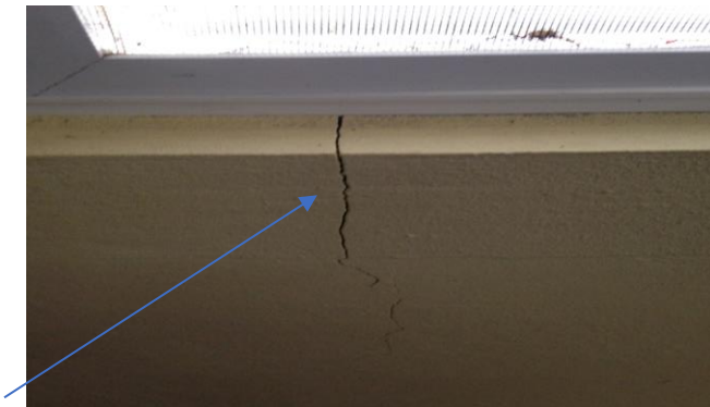
Crack in window in dining area begins on the inside under window frame, continues across the windowsill to the outside.
